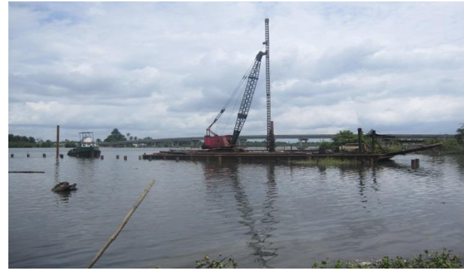
Uncompleted Jetty in Omadino, Warri South LGA, Delta State
