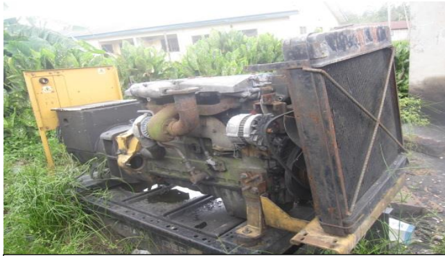
Non-functional generator in Ugbegugun-Escravos, Warri South West LGA, Delta State
